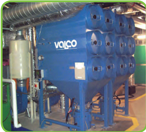
Cartridge filter with 60m 2 filter area (PTFE-membrane) and 60m 2 secure post-filter, filter system inside ATEX-zone 20
