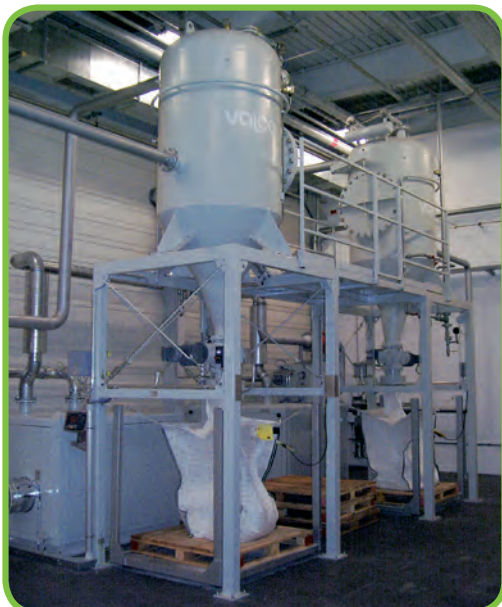
Central vacuum cleaning system in the automotive industry, explosion-proof, air volume of 2000 m 3 /h at 40 kPa vacuum.
